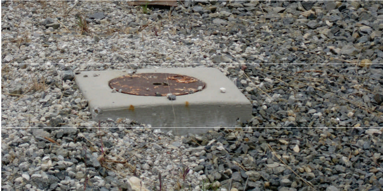
Tripping hazard, especially at night. Uneven communications box
