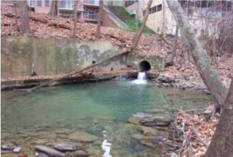
Another view of the outfall discharging into Soapstone Creek behind 4411 Connecticut Avenue, NW. Note also the other outfalls, and the discoloration of the water.
