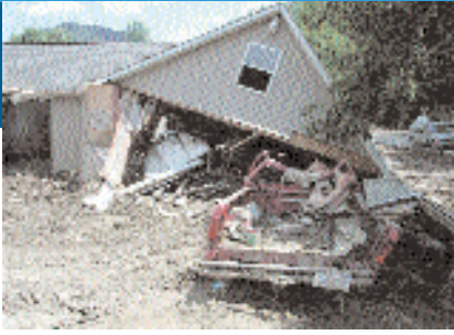
Flood damage caused in part by valley fills
