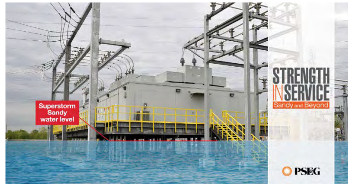
Image of PSE&G Raising Electric Infrastructure Above Superstorm Sandy Water Levels
