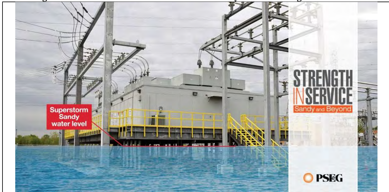
Figure 1. PSEG substation lifted above the 500-year storm surge flood level 16
