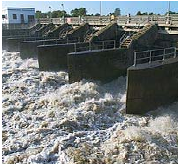
Figure 25. SFWMD structure S-80 discharging into the South Fork of the St. Lucie River. 63
