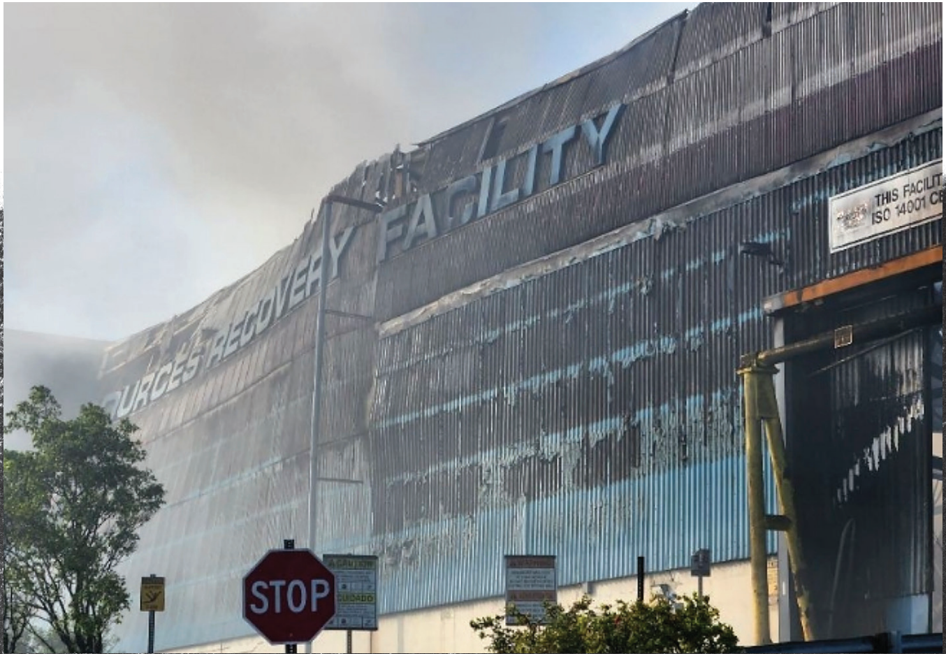
Exterior of the Miami-Dade County Resources Recovery Facility after a fire in February of 2023. Miami-Dade County Department of Environmental Resources Management
