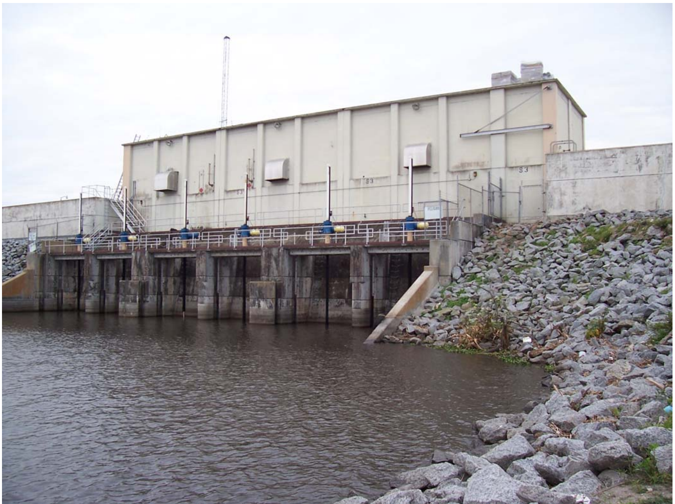
Massive S-3 pumping station that conveys polluted water into Lake Okeechobee.
