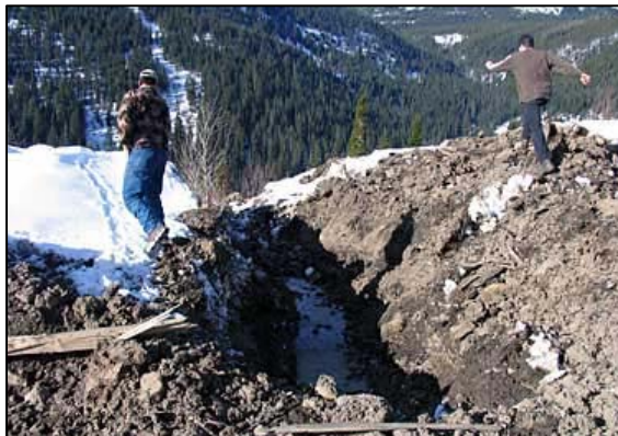
Mud drains from raw Cline culvert towards North Fork of Lodgepole Creek. Photo from Flathead Coalition.
