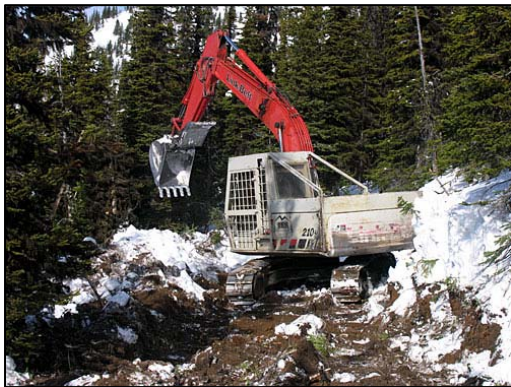
Cline Mining clearing roads in Foisey Creek drainage. Photo from Flathead Coalition.
