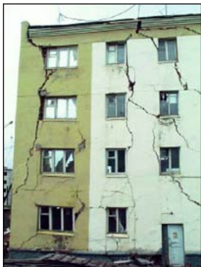
Cracking due to permafrost melting
