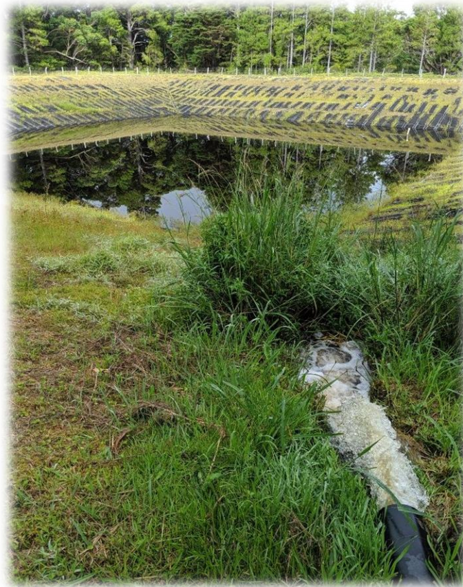
Recent dumping into old, pre-1998 reservoir
