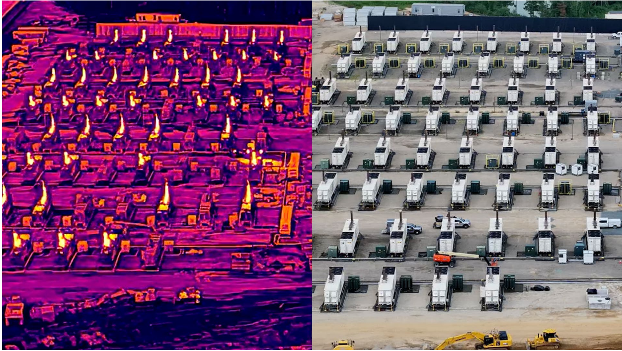
Figure 3: Fleet of 62 illegally operating gas-powered engines, each approximately 40ft long, 8ft wide, and 9.5ft tall. (Aug. 27, 2026, Evan Simon / Floodlight)
