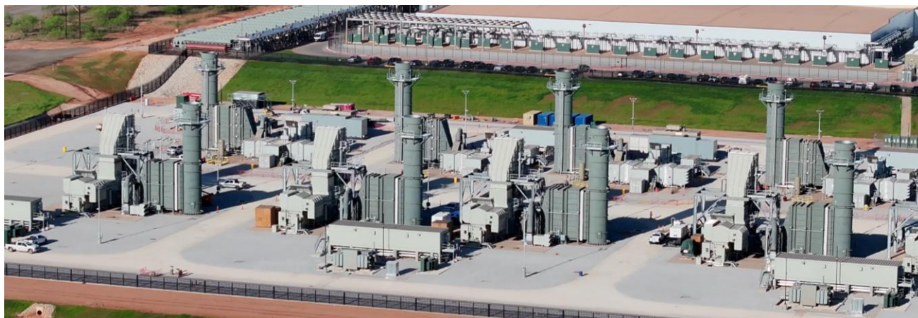
Simple cycle gas turbines at OpenAI’s campus in Abilene, TX (Evan Simon, Floodlight)
